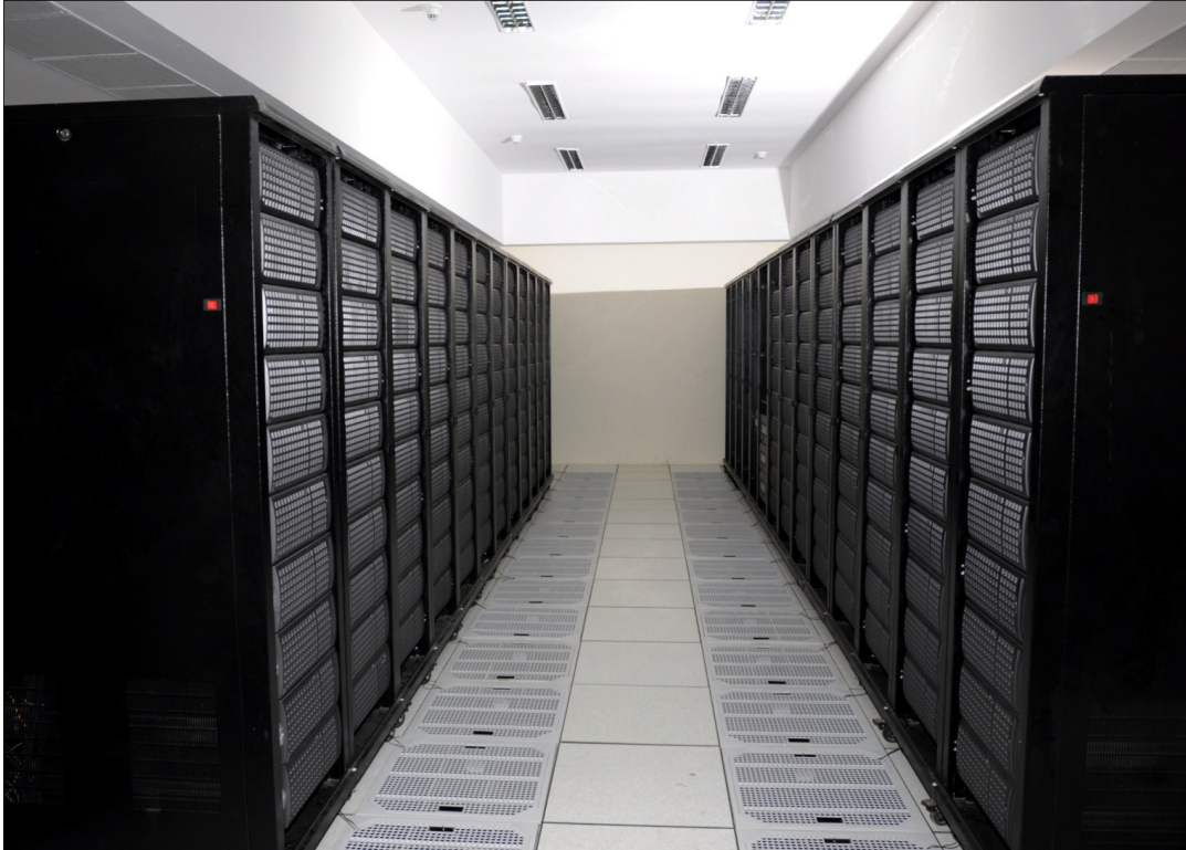
Figure 5.18 Photograph of SAGA supercomputing cluster ( www.ISRO.org )
